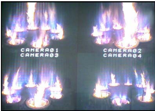
Monitor View of Fired Heater Burners
