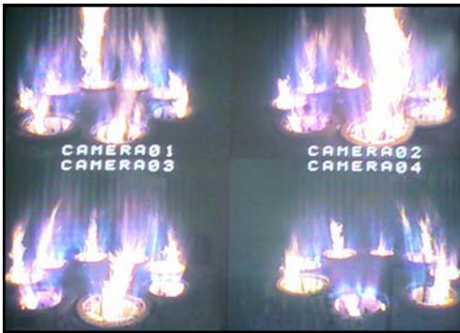
Monitor View of Fired Heater Burners
