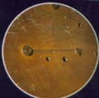
Actual photo taken through Lenox rigid borescope shows missing rivet on structural component.
