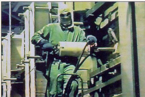
Fig. 1 Wearing fire-retardant gear, a technician inserts the periscope of the CCTV system into the regenerator chamber of a glass furnace to view checker packs used to regenerate heat during manufacture of glass.
