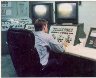
Control room operator views the fire inside two furnaces of the waste-to-energy plant operated by Montanay Power Corp. in Conshohocken, PA.
